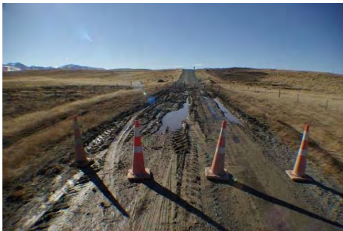
Braemar Road – Frost Heave July 2012
