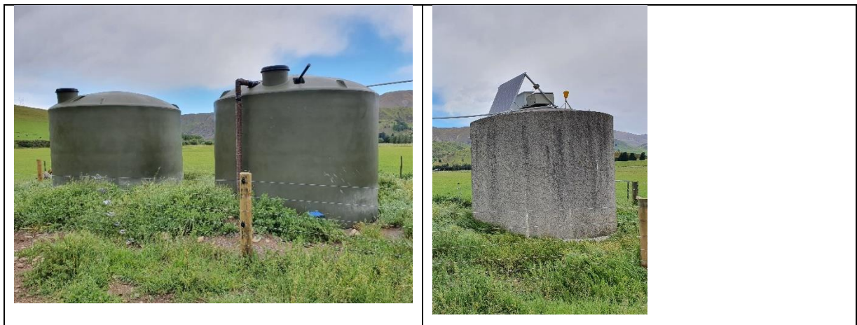
Figure 4-6 Burkes Pass Treated Water Storage Tanks
