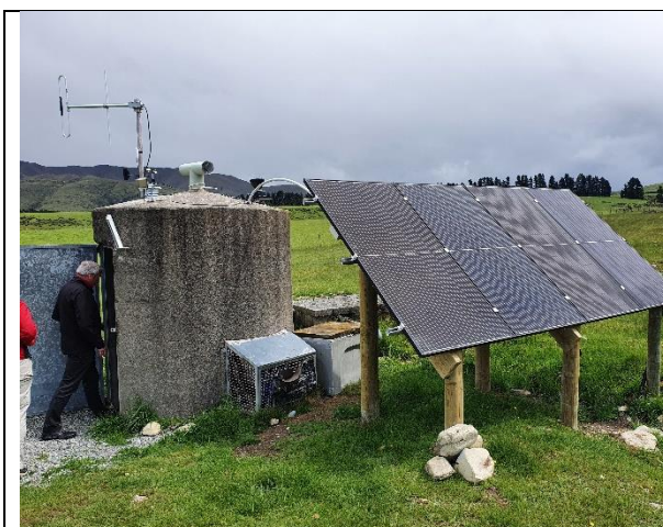
Treatment shed with solar panels
