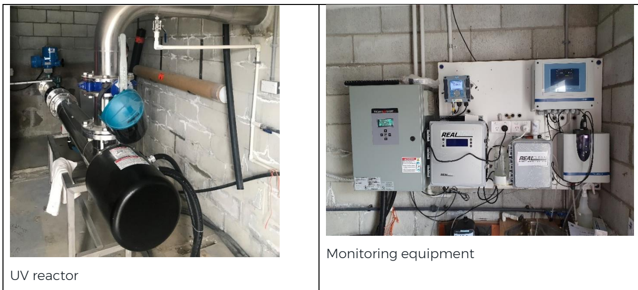
Figure 4-6 Tekapo/Takapō water supply UV treatment plant
