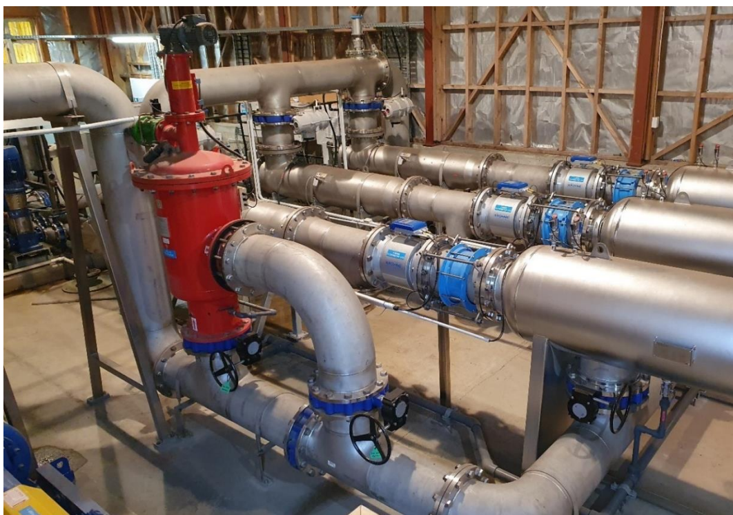
Figure 4-7 Twizel water treatment plant UV disinfection reactors
