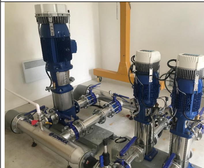
North West Arch pumps (boosting supply to The Drive subdivision)
