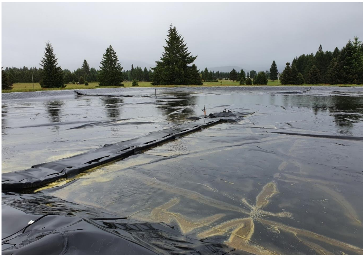
Figure 4-5 Raw water storage pond with HDPE liner and cover
