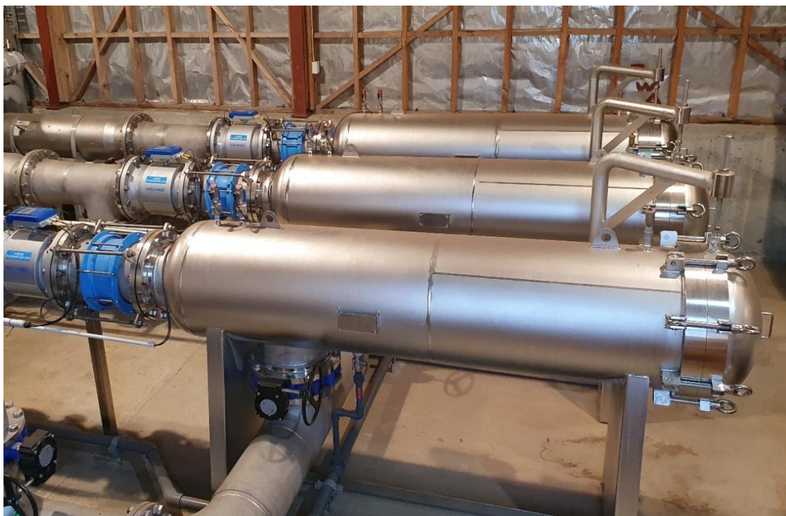
Figure 4-6 Twizel water treatment plant cartridge filters
