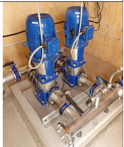
Pukaki Airport pumps
