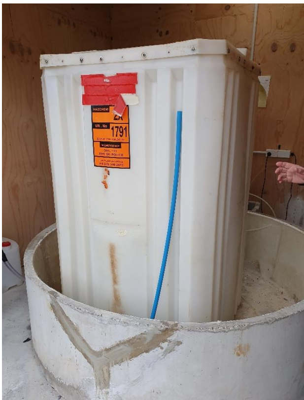
Figure 4-8 Twizel treatment plant hypochlorite dosing system
