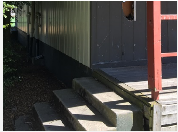
Photo 8. Secondary stairs without handrails
