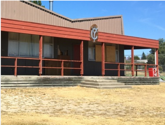
Photo 7. Main entrance stair without handrails
